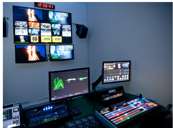
Fighting Irish digital media control room
